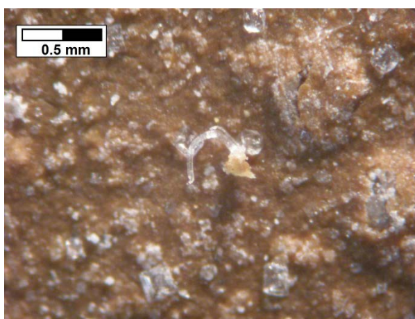
Figure 6 – Needlelike efflorescence causing spalling.
