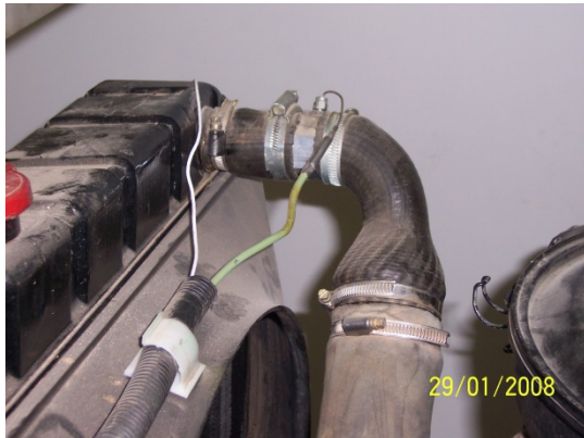
Figure 7: Inlet Radiator Temperature sensor
