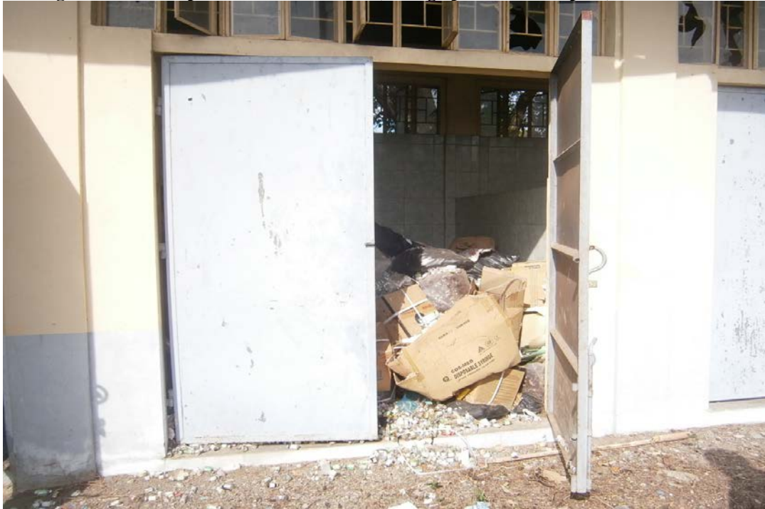
Figure 11. Old Disposal for Waste Water (Kalinga provincial Hospital)
