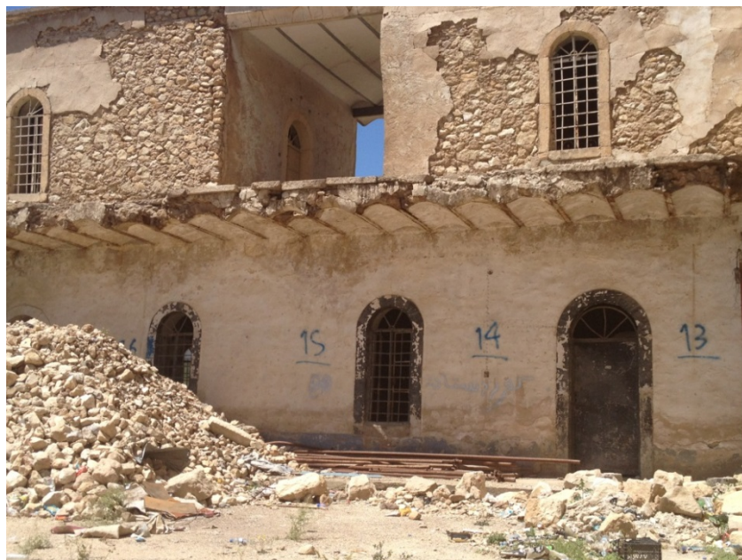
Fig. (7) and Fig. (8) show the poor condition of houses and services in old Akre. Source: Researcher
